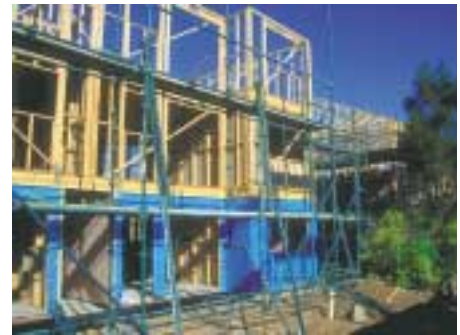
The first Australian MRTFC project under construction in 1995. The Lutwyche 3 Storey, Class 2 Project was the beginning of timber framed multi-residential construction.
